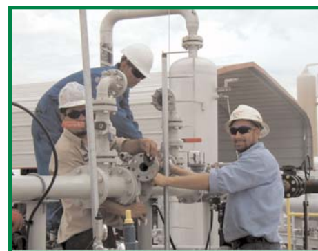
Installation of GHG Center flow monitoring equipment on the COMM EVRU system.
