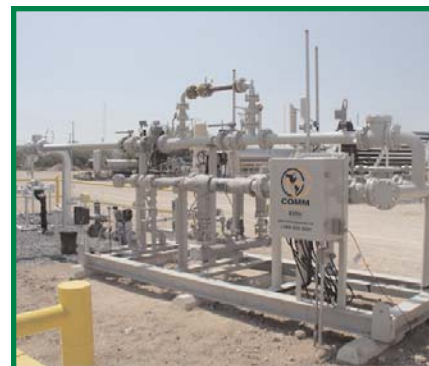
COMMA Engineering EVRU™ at the Total FinaElf Test Site in Texas.
