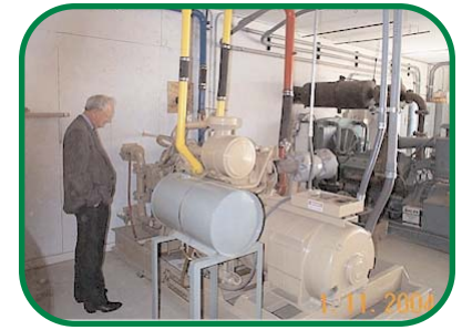
Biogas fueled engine-generator-CHP in use at a swine farm.
