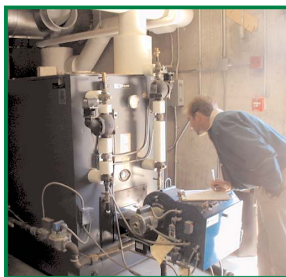
Existing boiler at Crouse Community Center that will be operated less due to the recovery of waste heat from the PowerWorks™.
