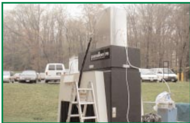
Honeywell Parallon® 75 kW Turbogenerator Test Site in College Park, MD
