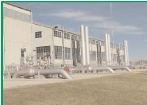
Typical Natural Gas Transmission Station in the U.S.
