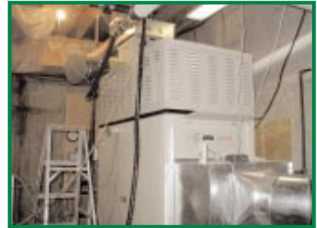
Mariah Heat PlusPower™ System Test Site in Calgary, Alberta, Canada
